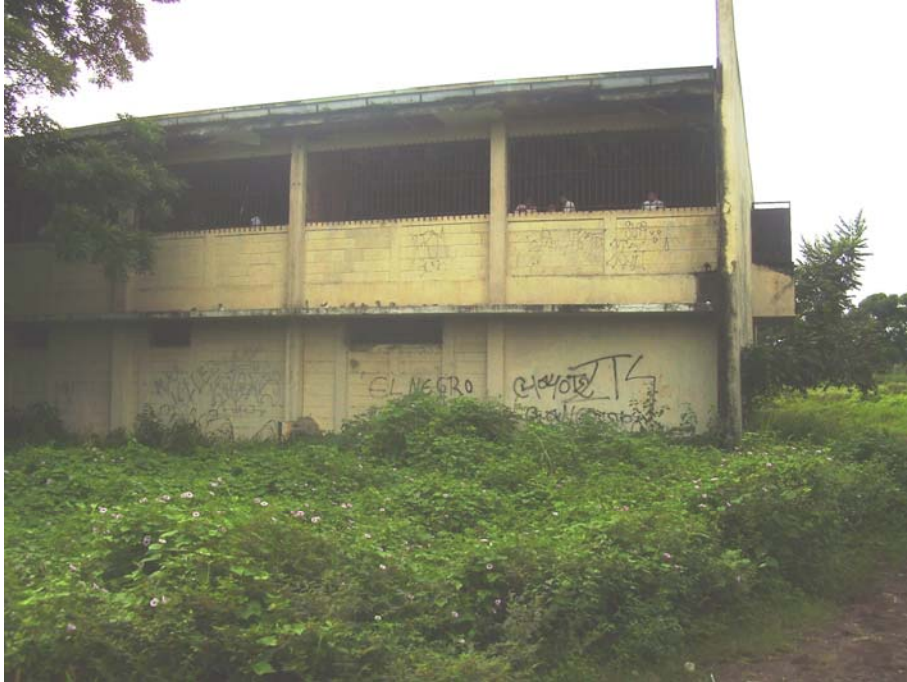
The grass and bushes around the building are very dangerous for students.
